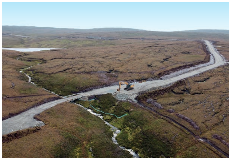
The wind farm track network is nearing its full geographical extent. This picture shows good progress being made to the south of Scallafield in the west.
