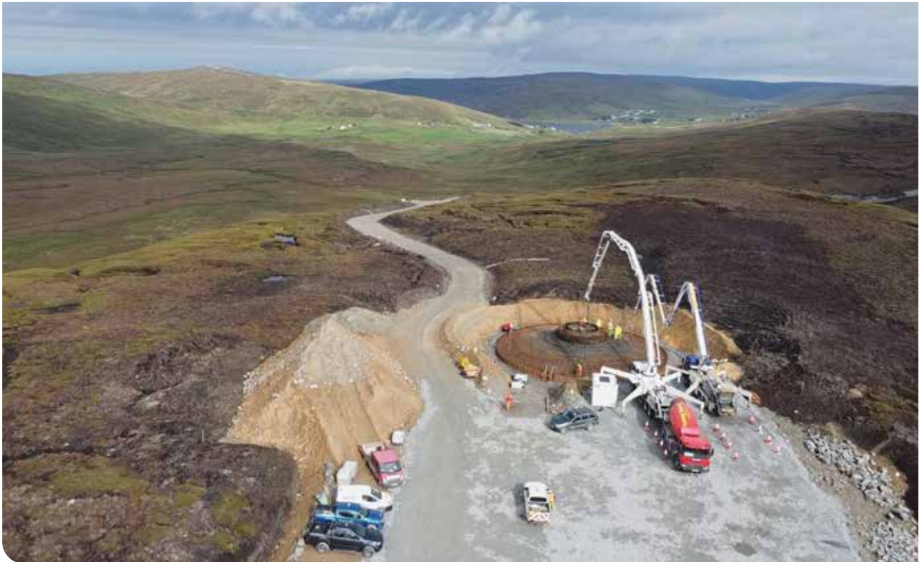
An all-day concrete pouring operation on the base of turbine K81 on the Mid Kame ridge.
