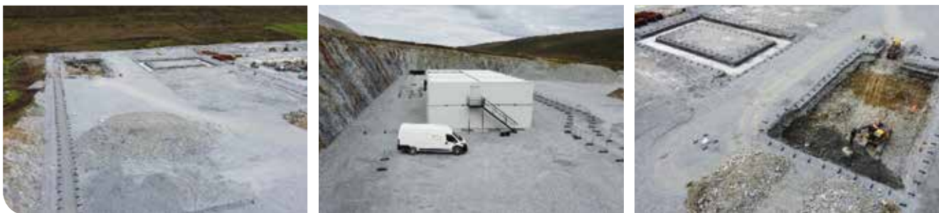
Work is now beginning on the wind farm AC substation on the Upper Kergord platform.
