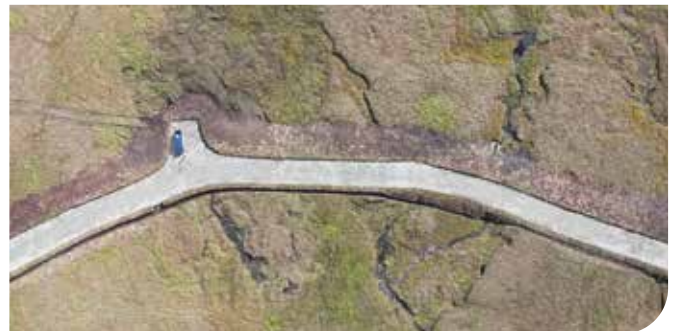
Careful road construction and high-quality verge reinstatement makes for a neat job which should knit into the landscape in the years to come.
