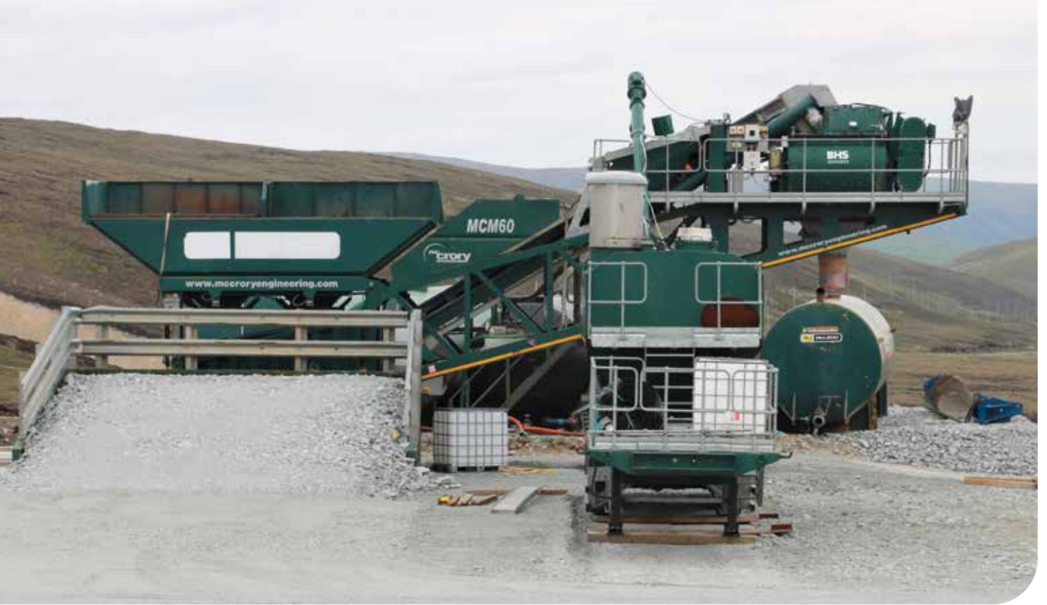
The first concrete batching plant in the new temporary North Compound, south of Voe.
