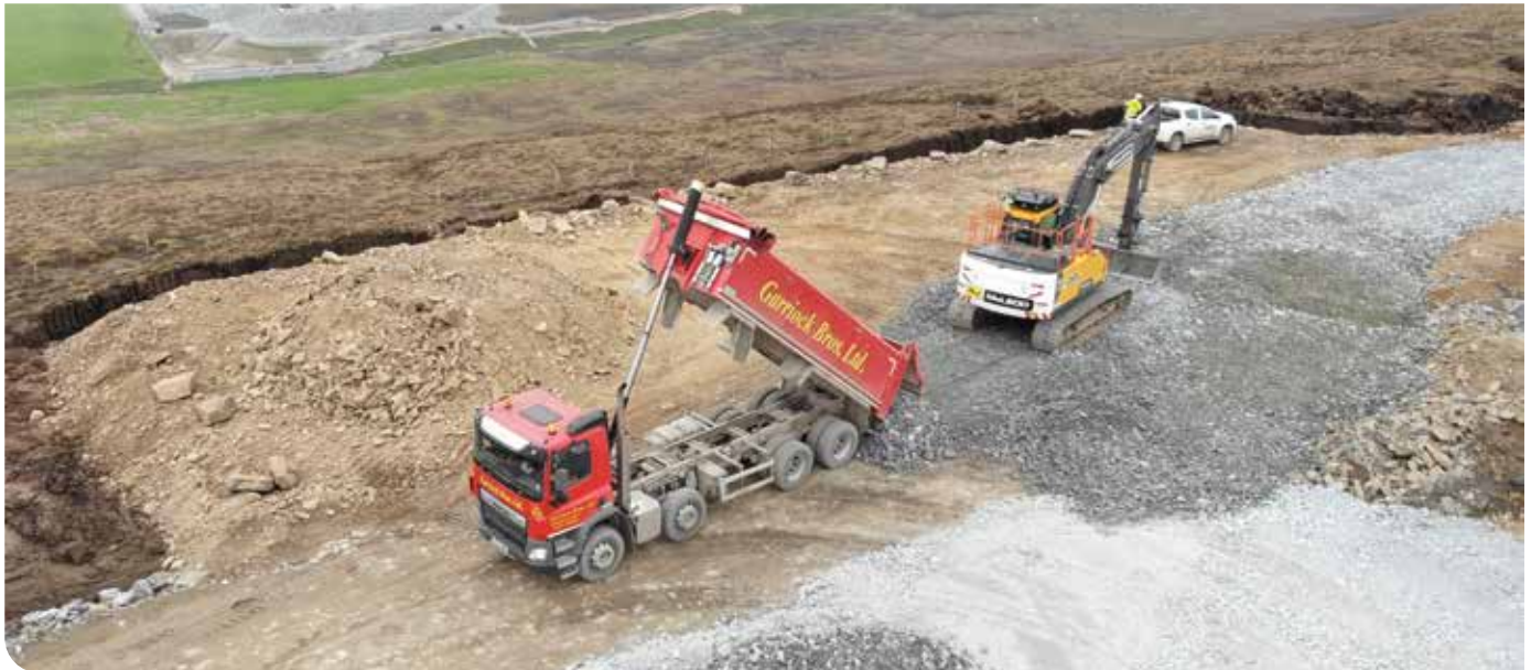
The capping layer on the Mid Kame track. The SSEN Transmission project site at Upper Kergord can be seen in the background.
