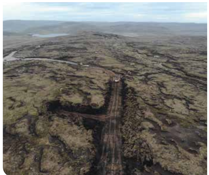
Much of the peat to the east of the Lang Kames is severely eroded, such as where this track is being built at Scar Quilse. The Loch of Voe can be seen in the distance.
