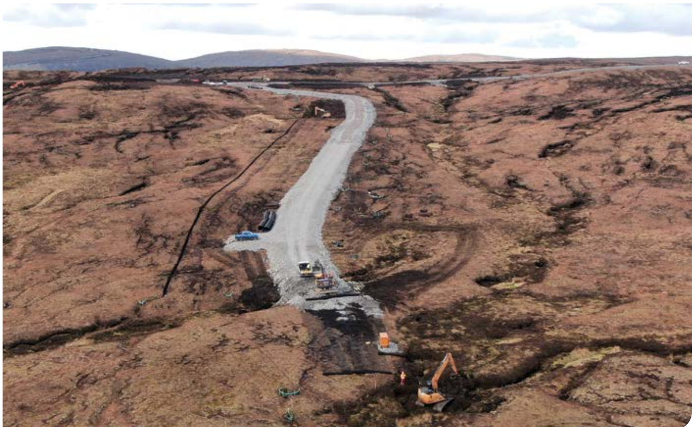
A floating access track to a turbine site above Catfirth in South Nesting.
