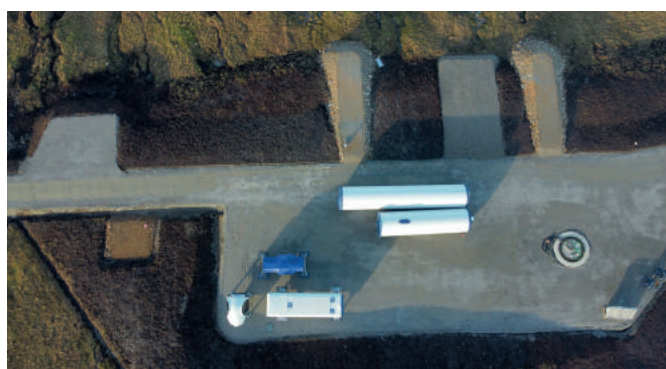
Backfill cable trenches allowing final capping and landscaping ahead of component deliveries.
