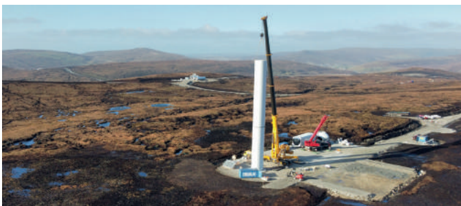
First two tower sections bolted into place, North Nesting. The first fully erected turbines are expected in April.
