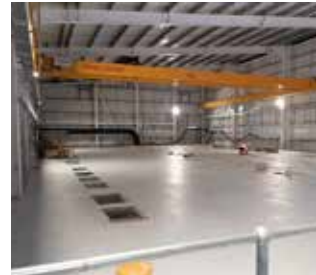
Protection & Control Panels Installed.
