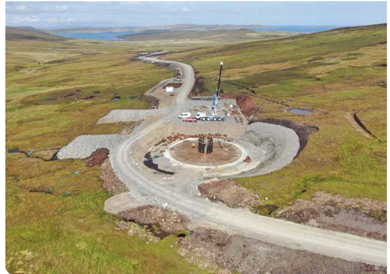
A turbine foundation anchor cage under construction near Dury, South Nesting, in preparation for concrete pouring. At the time of writing, around 80 bases have been poured and all remaining concrete pours will be in the South Nesting section of the site.
