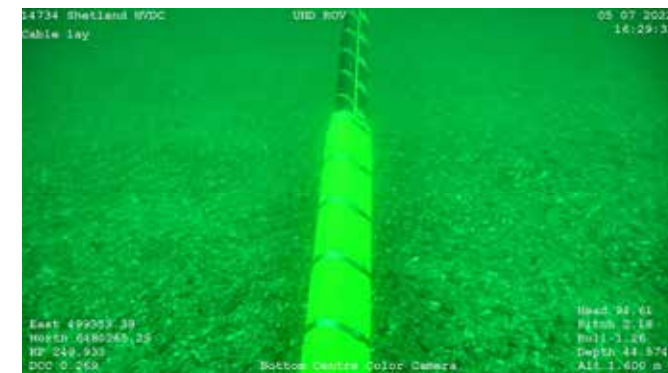
Cable Protection System (CPS) across the Horse Mussel Bed.
