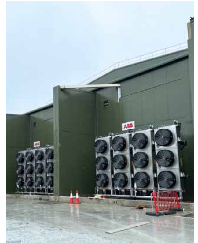
Completed transformer enclosures with cooling fans visible.
