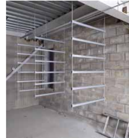
Containment brackets in Basement.
