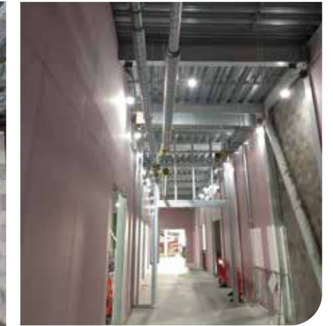
Ventilation 1st floor Services Building.
