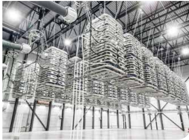
Hitachi Energy IGBT valves.
