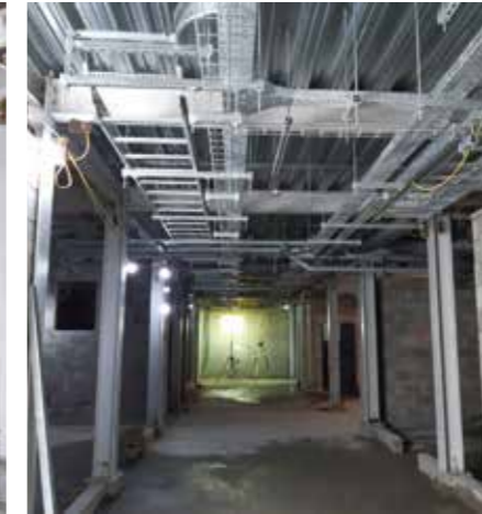
Power and Lighting containment.
