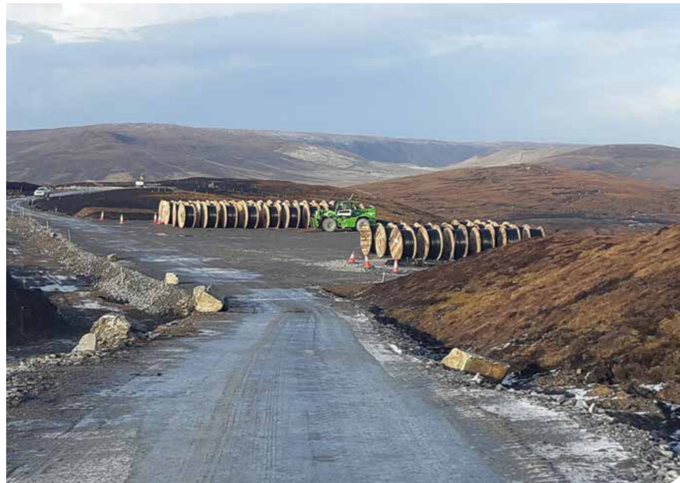
Cables deployed on Mid Kame ready for installation. Once cables are installed verge reinstatement can be completed to match the successful reinstatement shown on the right of the picture.
